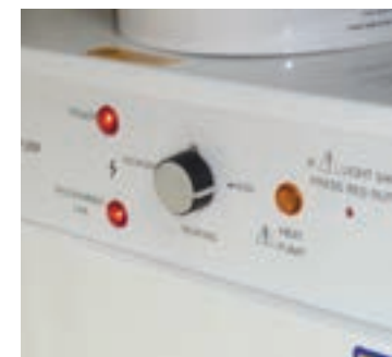
Some of the monitoring and controls equipment installed at House 60.
