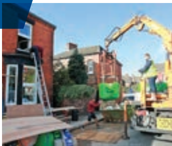
Lack of space on site caused difficulties on several projects including at House 69 (top). At House 85 (above) materials had to be stored on the road in front of the house.
