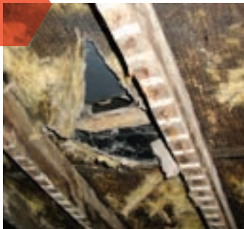
Problems uncovered by “systematic destruction” before the retrofit work began [North Belfast, case study 1, House 1, page 44].
